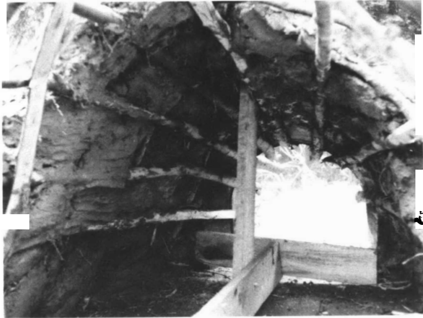
The bare framework begins to disappear under the clay vault Lise and Jean-François Blanchette Collection
